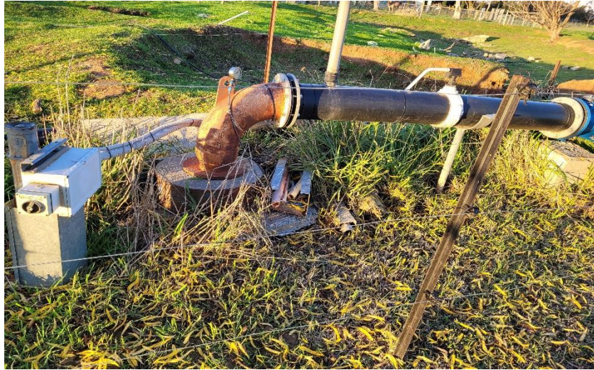
Pump/ bore site
